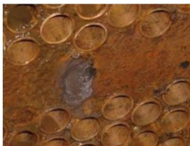
Microbiologically Induced Corrosion (MIC)
