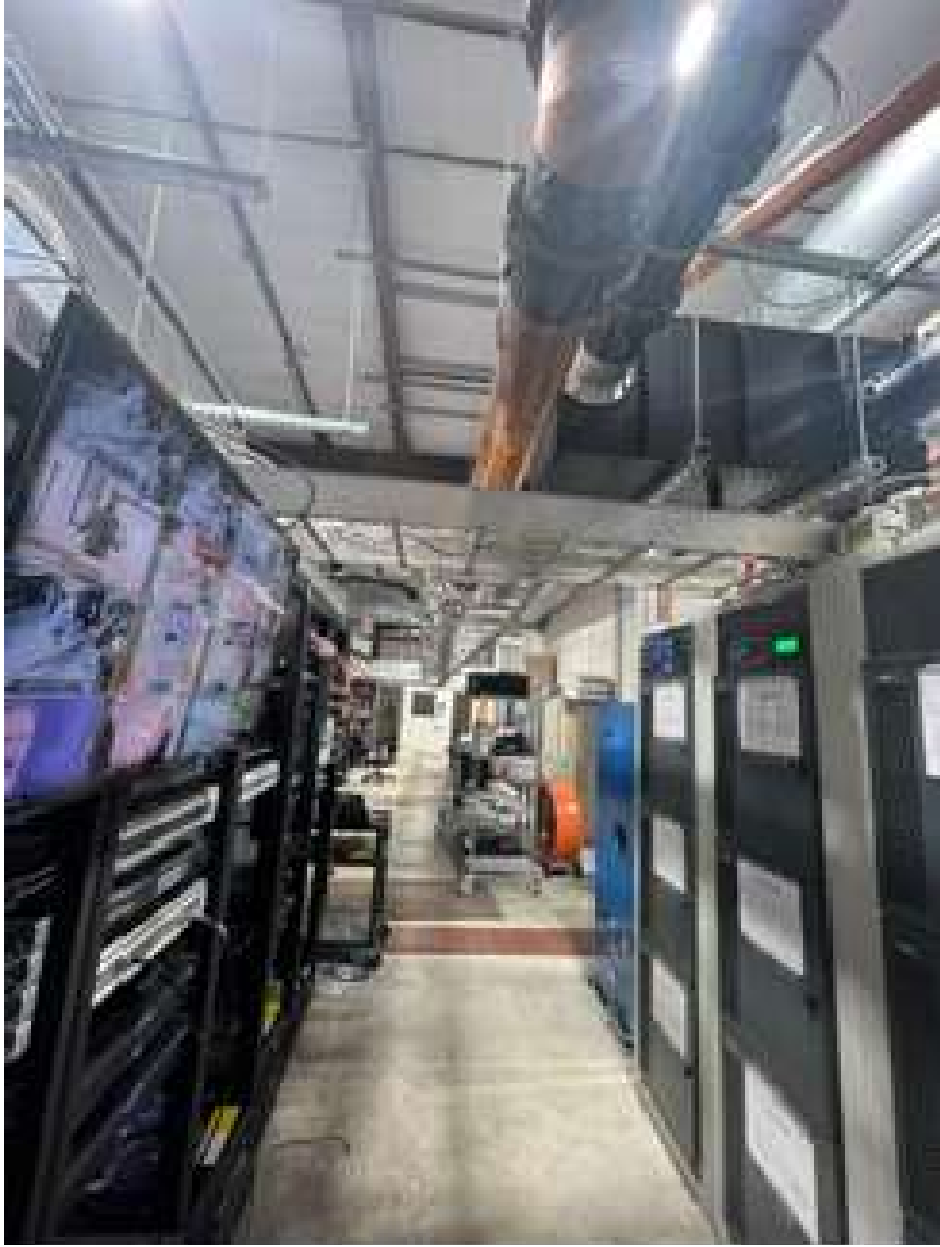
WUCF RACKS LEFT XMITTER RIGHT RACK TOP
