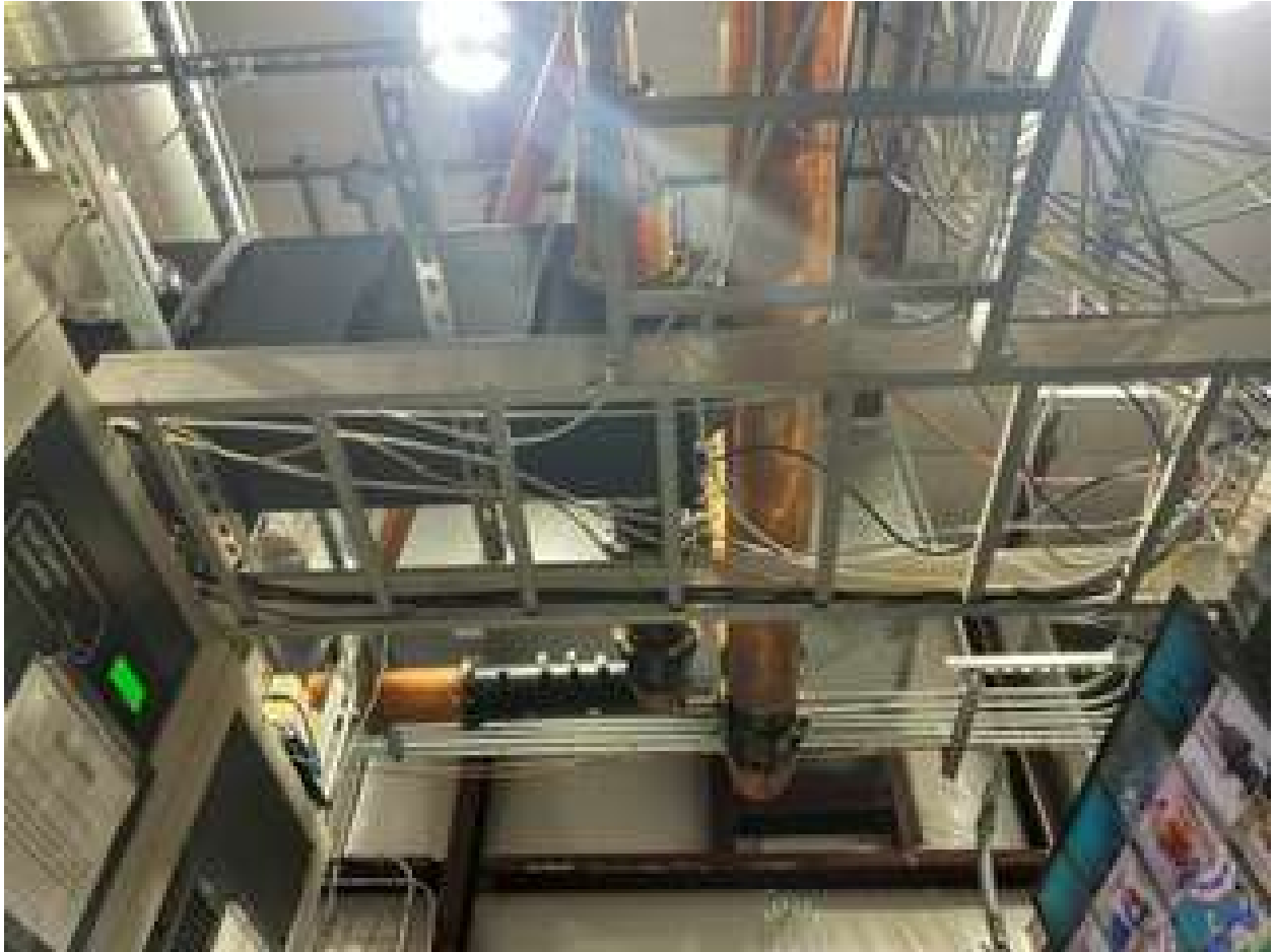
CABLE TRAY FROM RACK TO XMITTER
